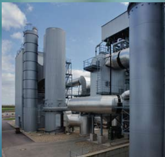
The exhaust gas treatment system at f | glass GmbH
